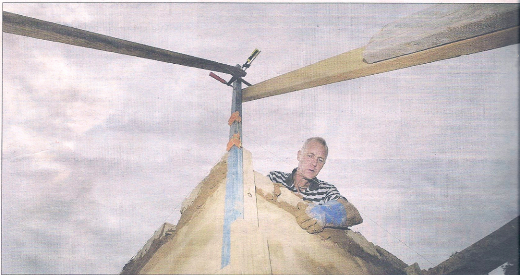
Mud bricklayer David Young works on a building at St Andrews, with a new study hoped to prove mudbrick buildings' energy efficiency.
